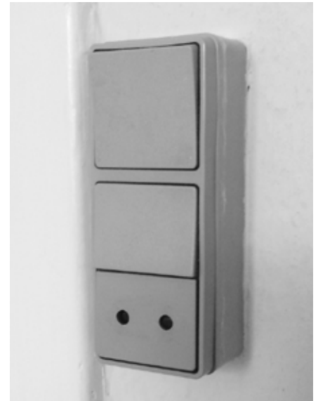
Figure 5. Danish light switch.
