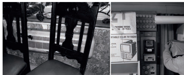
Figure 3a: A hidden air pump. Figure 3b: An electricity meter uncovered in the basement.
